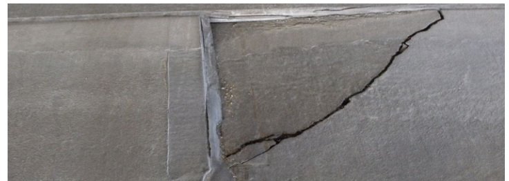
Example of damage caused by earthquake
