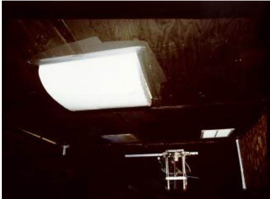
Figure 5.3.01 Total Air Distribution (TAD) Diffuser, and Velocity and Temperature Measuring Sensors
