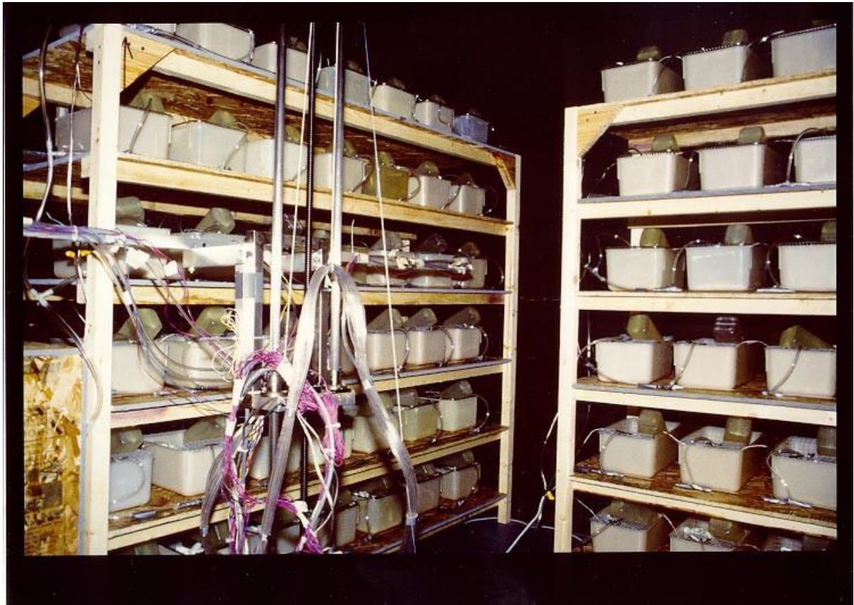
Figure 5.3.08 Typical Rack: Populated Room #3
