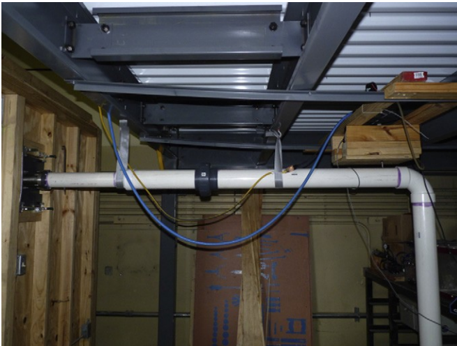
Fig. 2. Air inlet system e particulates were injected into this horizontal inlet pipe on the right hand side and the stainless steel inlet is shown fastened to the PTC on the left hand side.
