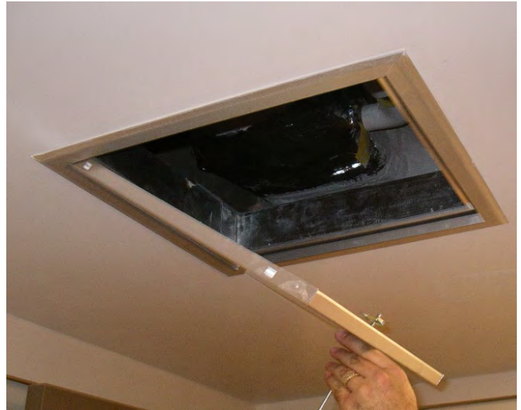
Ceiling Access Panel
