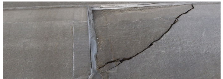
Example of damage caused by earthquake
