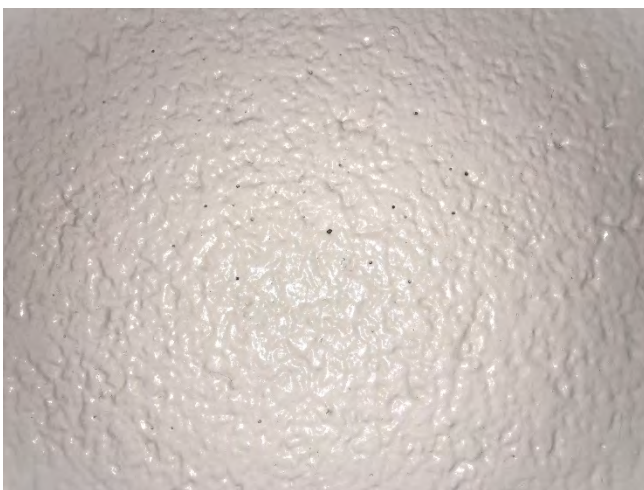
Figure 4.3.3.3.C: Epoxy paint with pinholes (Credit: NIH OD/ORS/Division of Veterinary Resources)
