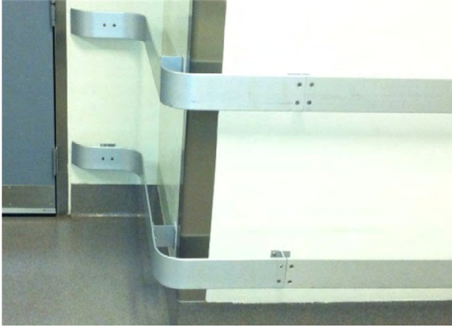
Figure 4.3.3.5: ARF wall protection
