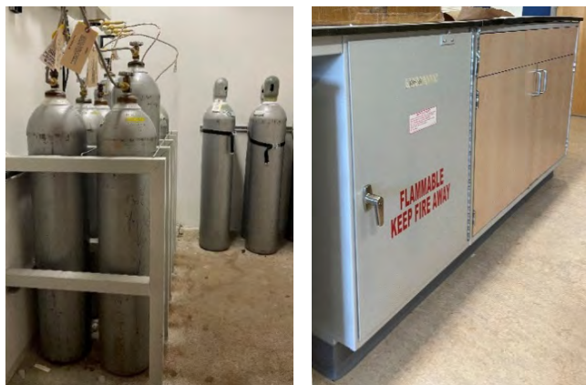
Figure 2.2.3.F: Gas cylinder restraints and Figure 2.2.3.G: Flammable storage cabinet
