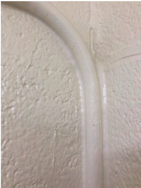
Figure 2.4.3.A: Wall-mounted conduit with sealant (Credit: NIH OD/ORS/Division of Veterinary Resources)
