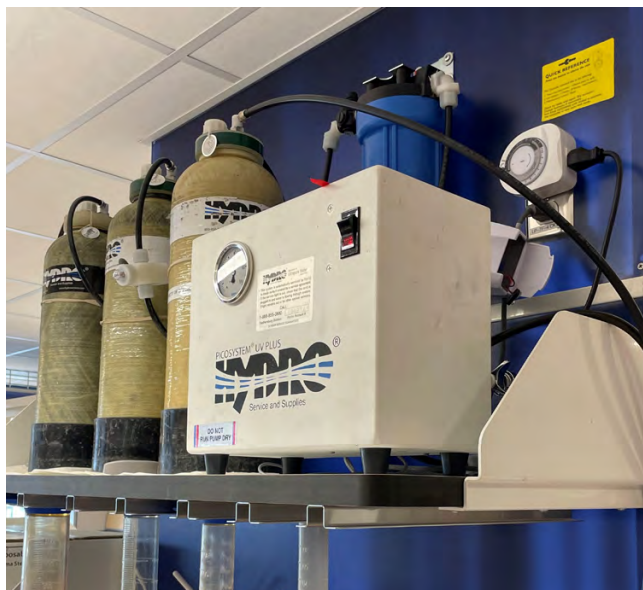
Figure 4.5.3: Water purification system with dedicated power receptacle.
