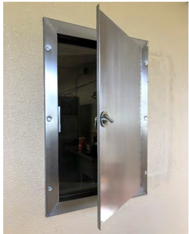
Figure 2.4.3.1: Stainless steel view window set into a fiber-reinforced plastic animal holding room door (Credit: NIH OD/ORS/Division of Veterinary Resources)
