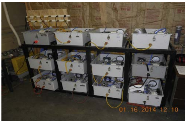
Fig. 4. General view of the 12 circulating air pumps that were connected to the 12 room air samplers. The air pumps were installed outside the PTC.
