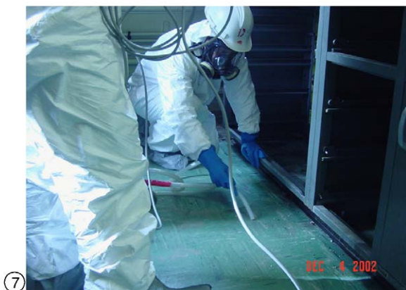
Figures 6 and 7. Cleaning Up Mercury Spilled from Casework During Laboratory Decommissioning Project.
